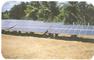
50KWp PV Power Plant at Neil Island, Andaman & Nicobar
