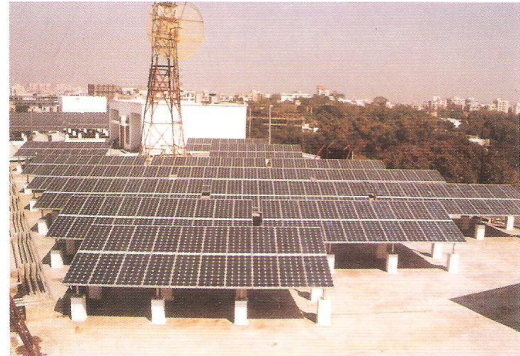
100 KWp SPV Grid Interactive Power Plant at APTRANSCO, Hyderabad
