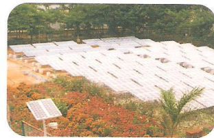
30 KWp grid interactive system ESD, BHEL, Bangalore
